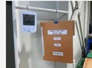
Installation of Temperature and Humidity Monitors
